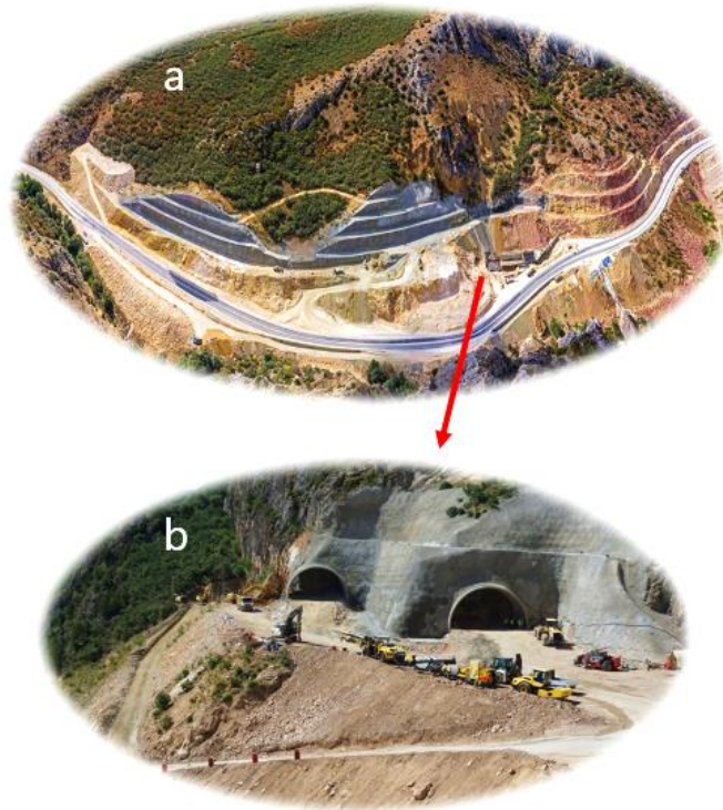
Figure 14. Tunnel entrances (a) starting from the steep slopes of Kırkdilim Canyon are constructed as right and left tubes (b). 33
