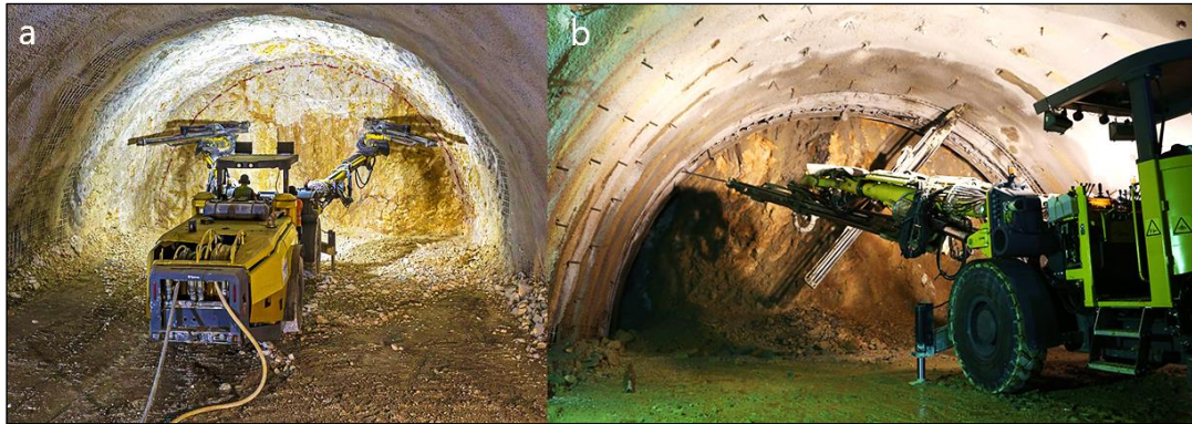
Figure 13. A view from double (a) and single (b) arm excavators digging Kirkdilim tunnels 32
